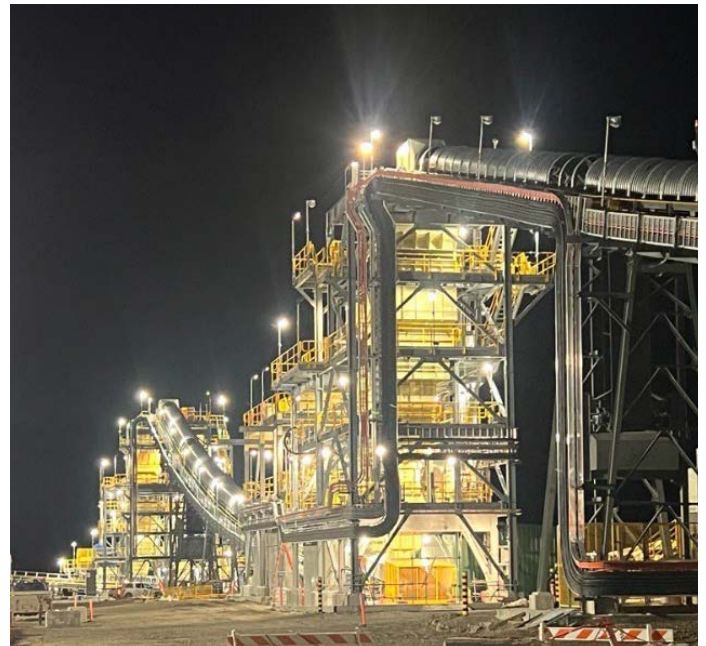
First ore was fed through the processing facility's crushing circuits in November 2024.
