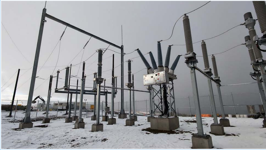
The 135-kilometre long 225kV transmission line between the Blackwater Mine and BC Hydro's Glenannan substation is complete and was successfully energized with renewable grid power on October 8, 2024.
