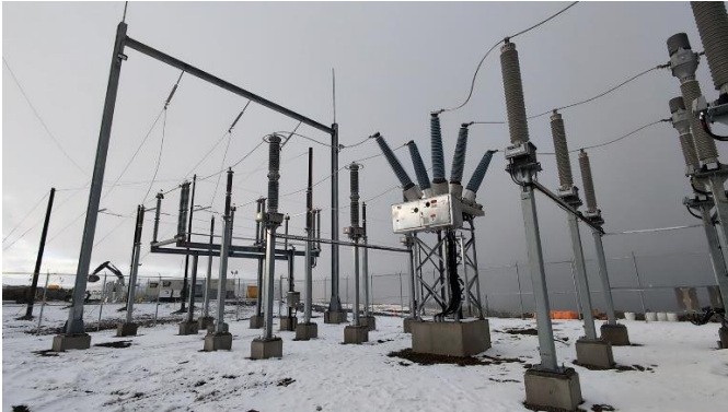
Blackwater 225kV substation
