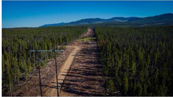
Transmission line to BC Hydro grid
