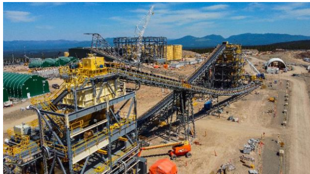
Tertiary crusher, conveyors & screening station
