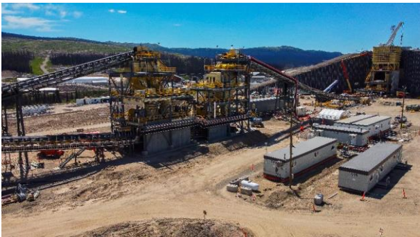
Secondary & tertiary crushers and conveyors
