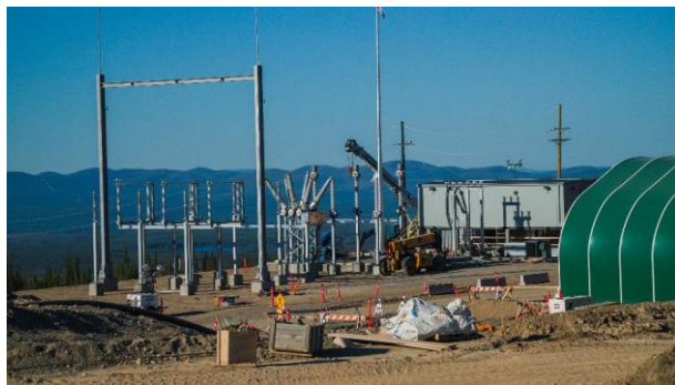
25 kV Electrical substation
